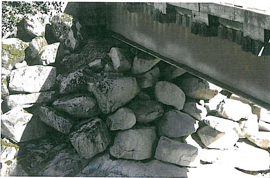
CK-2271 Left Rip Rap
